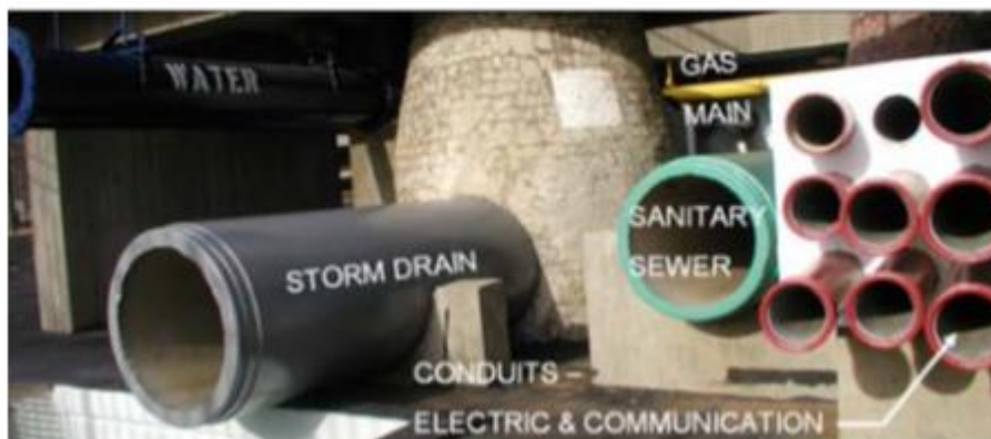
Figure 31: The need to know horizontal and vertical positions & type, size and location of existing subsurface utilities
